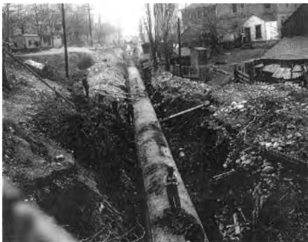
Figure 2 – Entombment of City Creek Canyon Stream circa 1909. U.S. Army Corp. of Engineers. From Love, ftn 22 infra .
