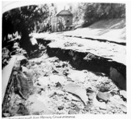
Figure 6 – Twelve Foot Deep Surface Failure North of Ottinger Hall and 400 feet north of proposed Well site, looking south, June 9, 1983. Salt Tribune. 1983. Spirit of Survival: Utah Floods of 1983.
